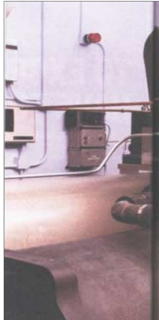
Photo courtesy of The Trane Company
